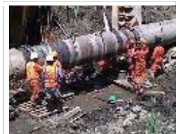
The tie-in between the onshore and offshore pipelines of the PNG LNG project took place in December, 2012. Image courtesy of Exxon.
